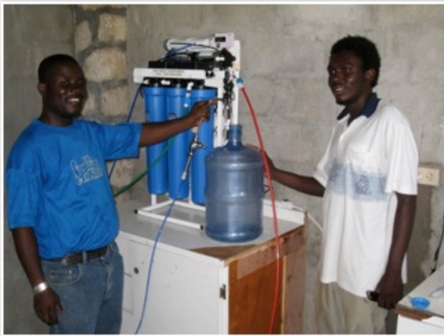
The water treatment system installed at The New Horizons School.
