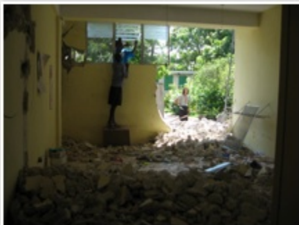
One of Sue's broken walls.
